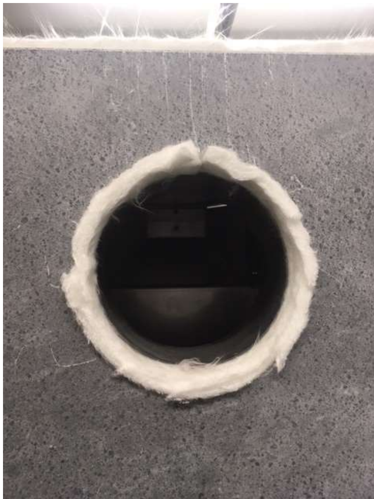
Back side chimney connection
