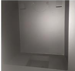
1. Clean fire chamber.
